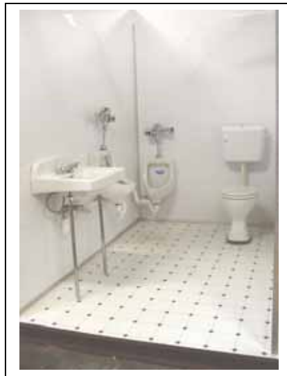
Fig. 8 ADA Unit With Auto Flushing Urinals
