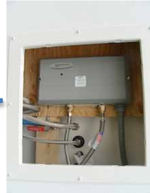
Tankless Hot Water Requires 220 V
