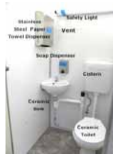
Interior Labeled View
