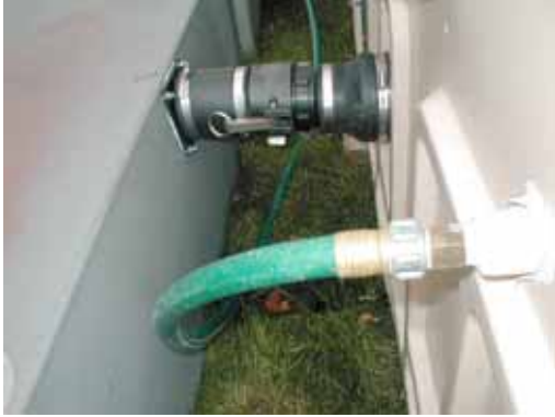
Holding Tank & Garden Hose
