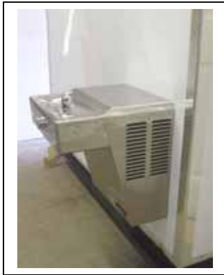
Cold Water Drinking Fountain
