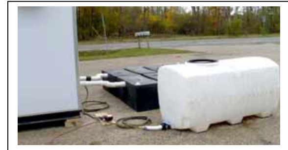
Holding Tank with Pressurized Water Tank
